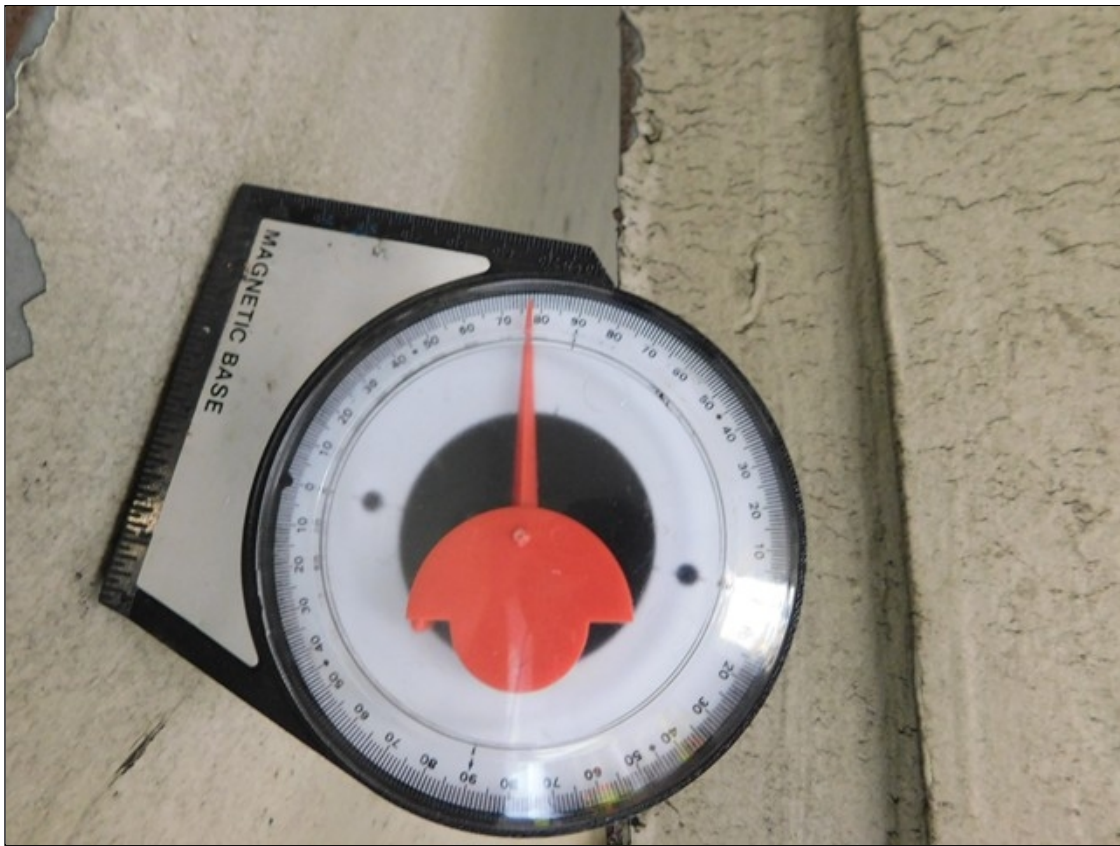
Span 2 Beam 10: BEAM 10 WEB IS OUT OF PLUMB 12 DEGREES AT 15 INCHES FROM THE BOTTOM FLANGE AND 16 DEGREES AT THE BOTTOM FLANGE FOR 25 FEET LONG STARTING AT BENT 1. A PRIORITY ACTION REQUEST IS BEING ISSUED FOR THIS BEAM.
