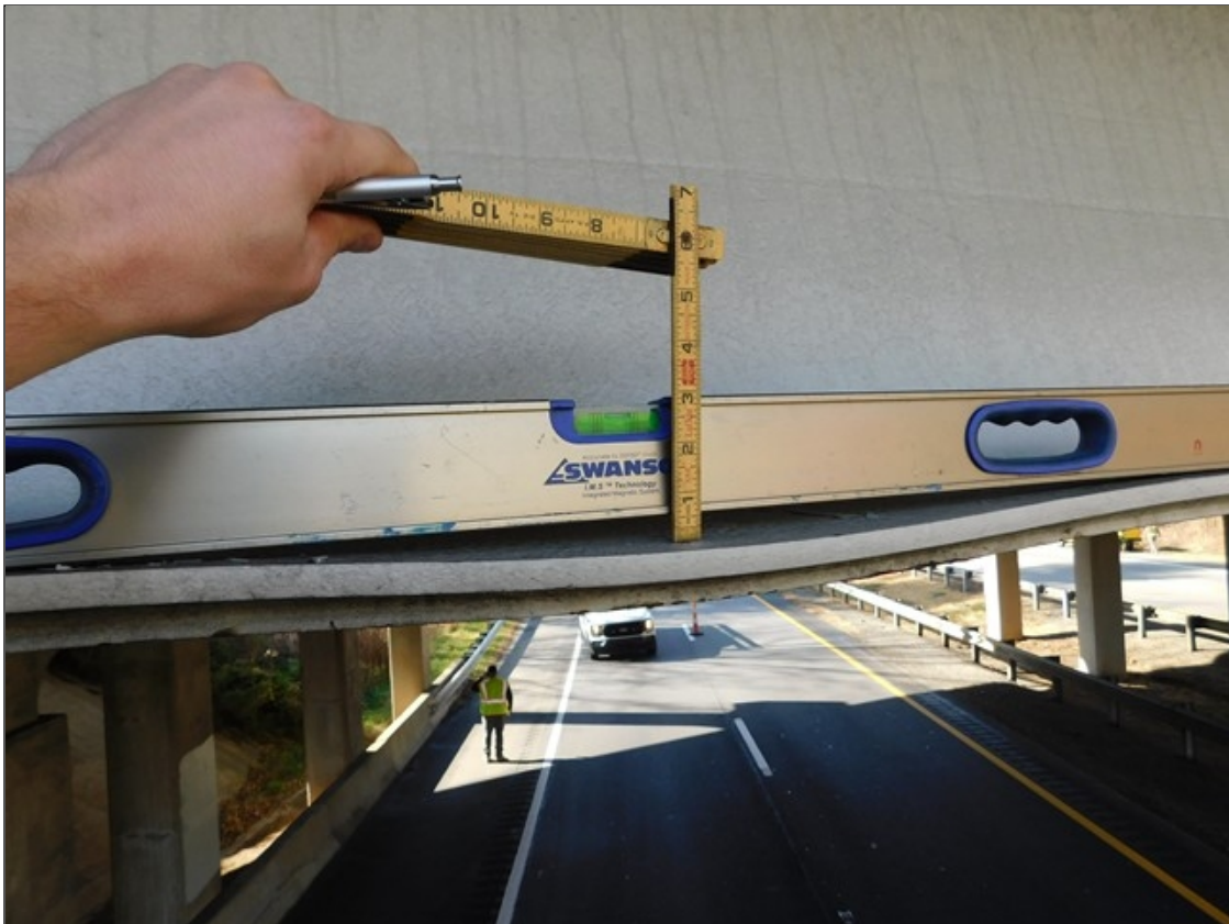
Span 2 Beam 10: BEAM 10 LEFT BOTTOM FLANGE IS BENT DOWNWARD 0.5 INCH FOR 28 INCHES LONG AT 15.2 FEET FROM BENT 1. OVERLAPPING QUANTITY.
