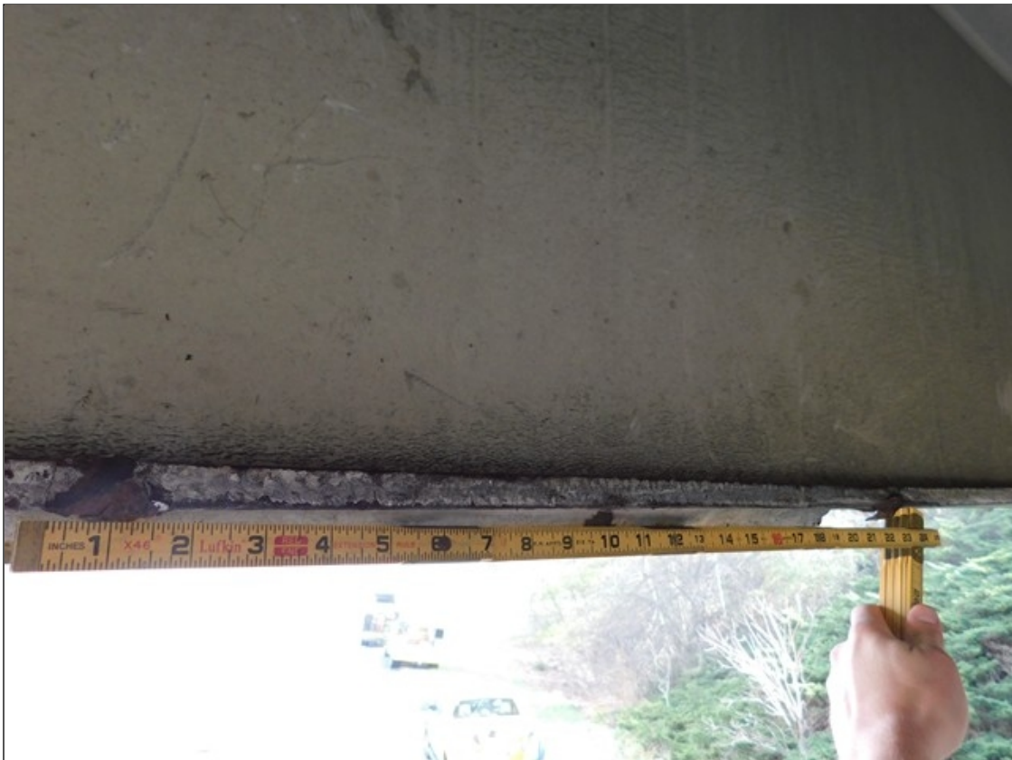
Span 2 Beam 10: LEFT EDGE OF THE BOTTOM FLANGE HAS A 1 INCH DIAMETER x 0.25 INCH DEEP GOUGE AT 11.1 FEET FROM BENT 1 AND A 1 INCH DIAMETER x 0.375 DEEP GOUGE AT 12.8 FEET FROM BENT 1.
