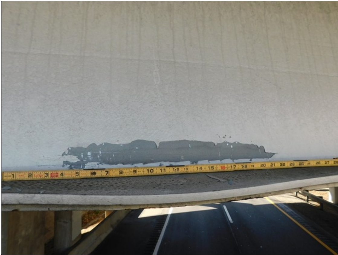
Span 2 Beam 10 - Protective System: PAINT HAS CHIPPED OFF OF THE RIGHT LOWER WEB 2.5 INCHES HIGH x 28 INCHES LONG AT 15 FEET FROM BENT 1.
