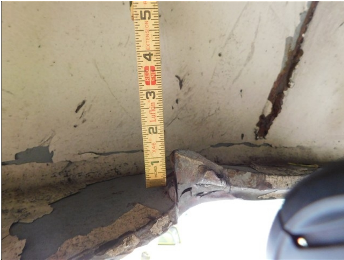
Span 2 Beam 10: BEAM 10 BOTTOM FLANGE IS BENT UPWARDS 4 INCHES x 28 INCHES LONG x 8 INCHES WIDE STARTING AT 15 FEET FROM BENT 1. THERE IS A 1 INCH LONG TEAR IN THE LEFT EDGE OF THE FLANGE. A PRIORITY ACTION REQUEST IS BEING ISSUED FOR THIS BEAM.
