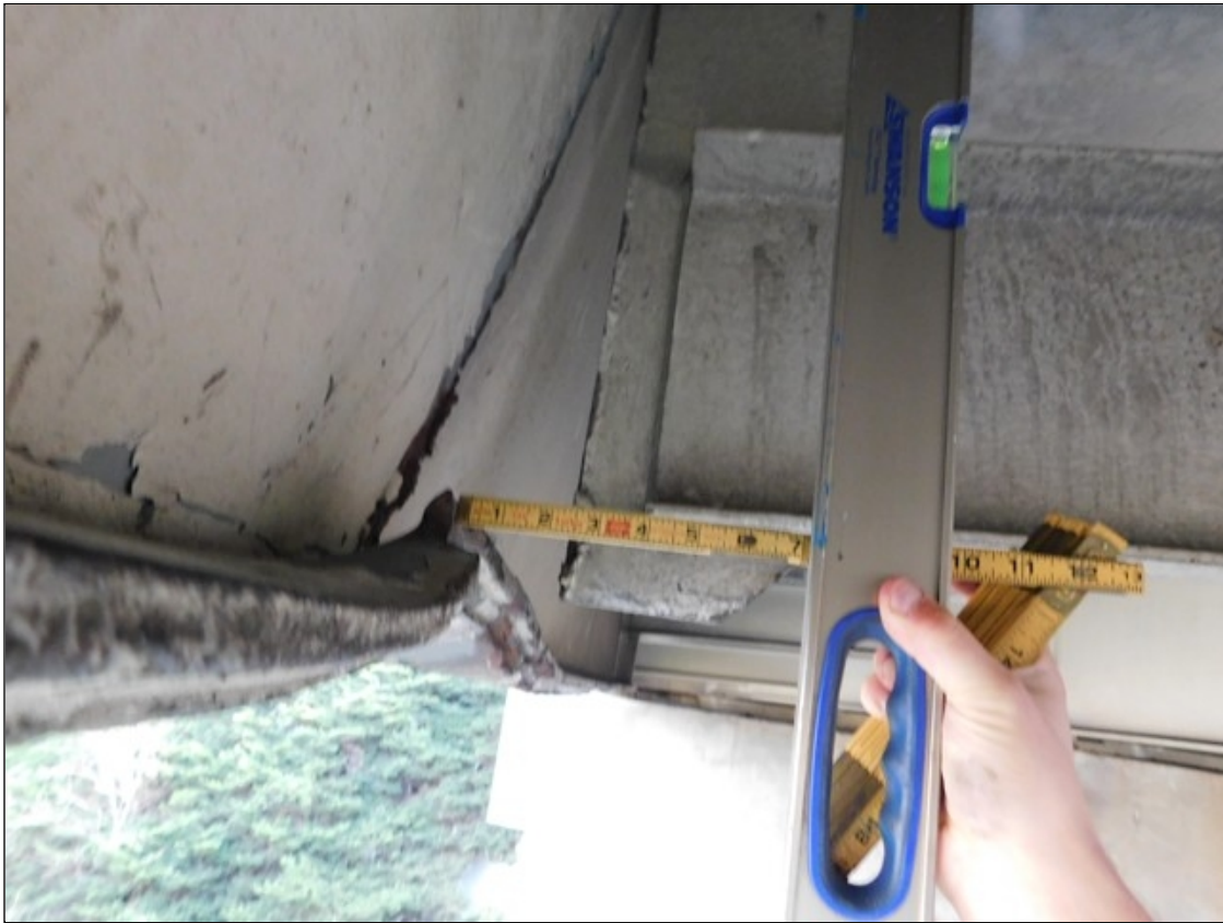
Span 2 Beam 10: BEAM 10 IS BENT WESTWARD FOR UP TO 7 INCHES x 25 FEET LONG STARTING AT BENT 1.
