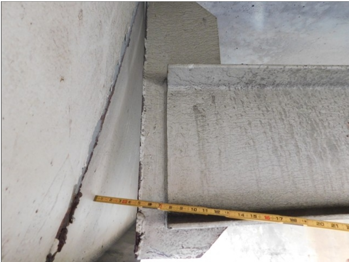
Span 2 Beam 10: SPAN 2, BAY 9, DIAPHRAGM 2 IS COMPLETELY SEPARATED FROM BEAM 10 AND IS SAGGING 1 INCH. A PRIORITY ACTION REQUEST IS BEING ISSUED FOR THIS DIAPHRAGM.
