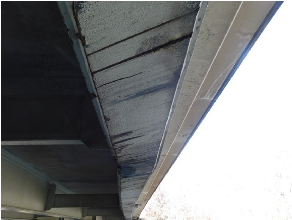
Span 2 Beam 10 - Protective System: BEAM 10 BOTTOM FLANGE HAS NUMEROUS SCRAPES ON THE UNDERSIDE OF THE BOTTOM FLANGE.
