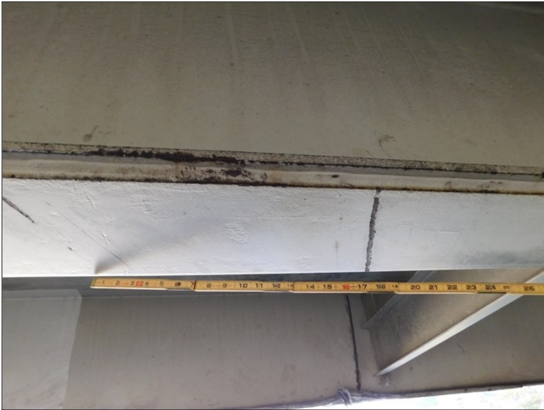
Span 2 Beam 9: SCATTERED SCRAPES ON BOTTOM FLANGE AT 16.2 FEET FROM BENT 1
