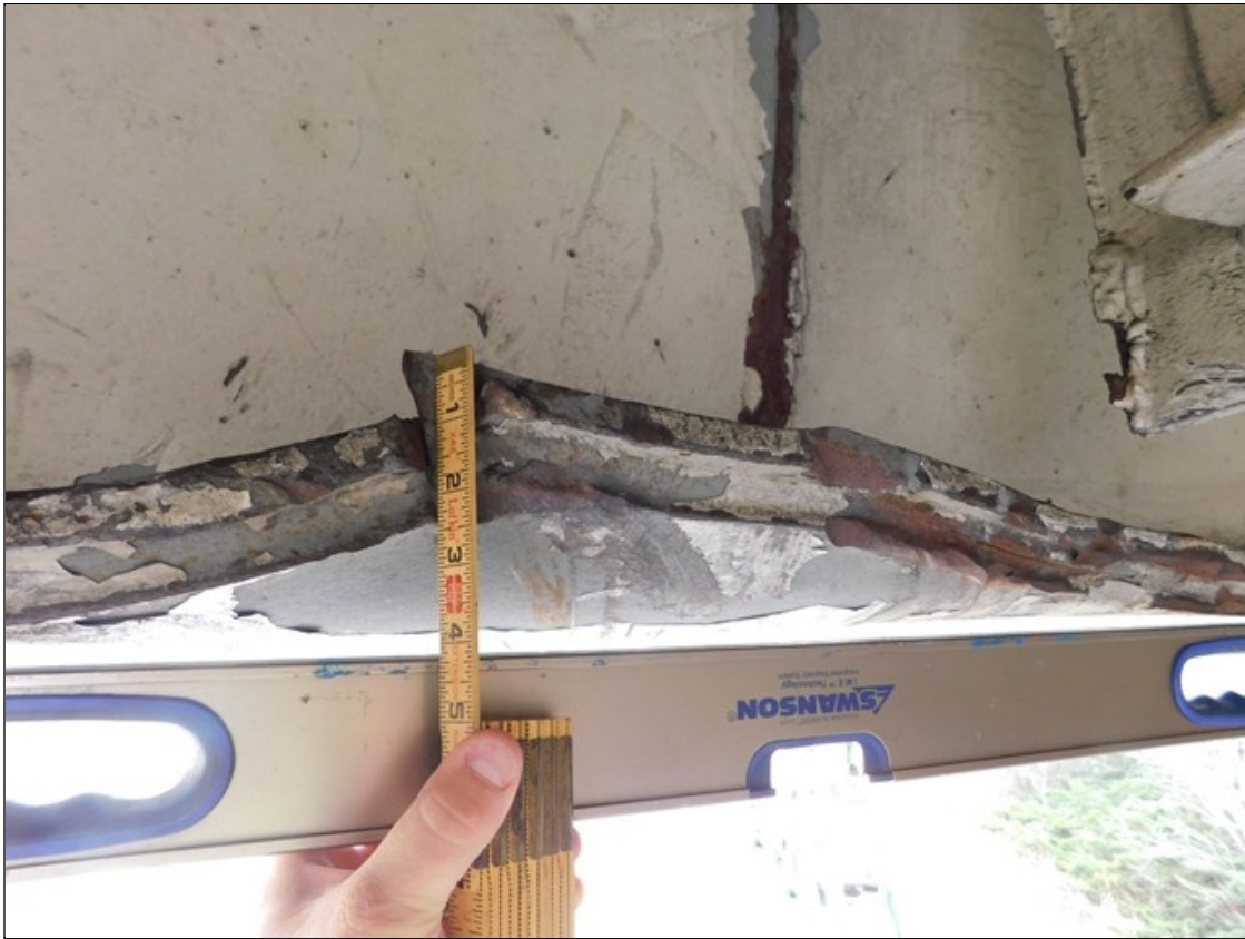
Span 2 Beam 10: BEAM 10 BOTTOM FLANGE IS BENT UPWARDS 4 INCHES x 28 INCHES LONG x 8 INCHES WIDE STARTING AT 15 FEET FROM BENT 1. THERE IE A 1 INCH LONG TEAR IN THE LEFT EDGE OF THE FLANGE. A PRIORITY ACTION REQUEST IS BEING ISSUED FOR THIS BEAM.
